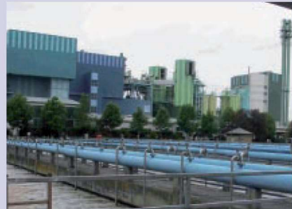
Measuring of the fluid and gas flow for the sewage treatment are primary tasks
